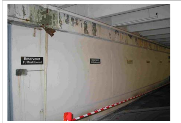
Fig. 12. Leaking of water and de-icing salts cause scaling of coating.
