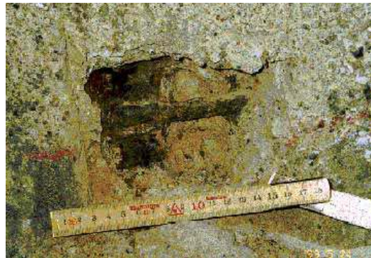
Fig. 4 Corroding reinforcement. Cross section loss : 1-2 mm
