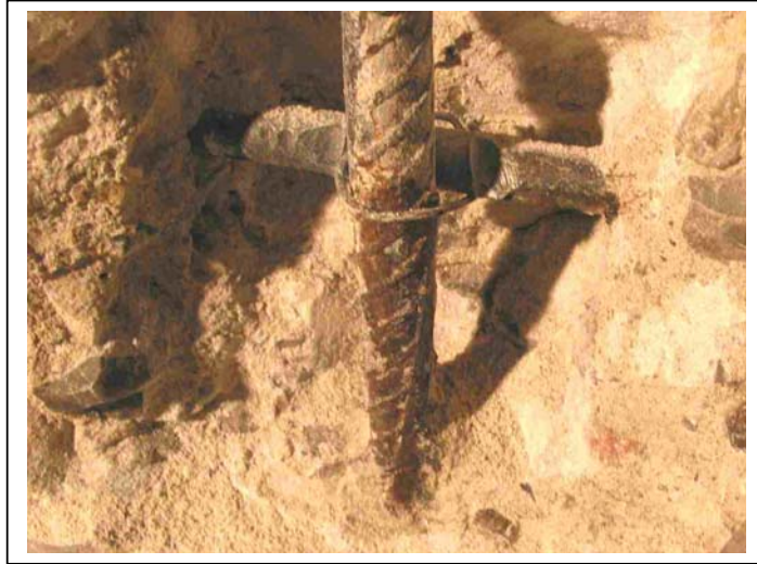
Fig.14. Exposed reinforcement at floor level in car park wall where HCP show very low values.
