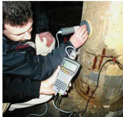
GalvaPulse testing in progress for corrosion activity of a heavily corroded column
