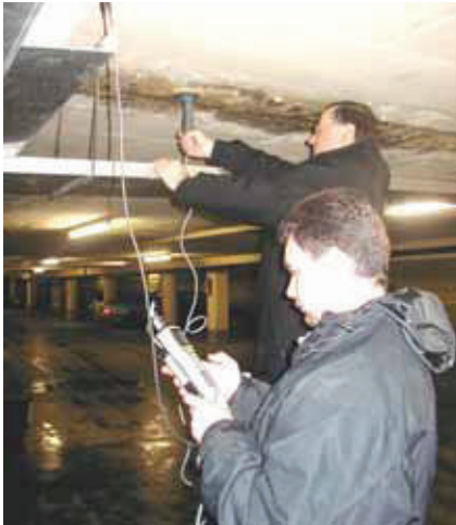
GalvaPulse corrosion rate measurement at a leaking joint
