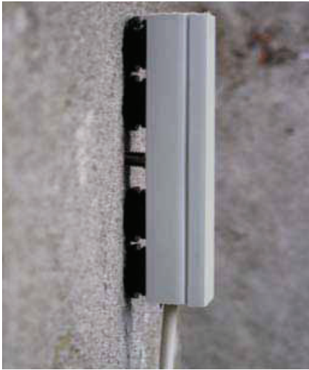
The CorroEye Mark I sensor installed on a vertical surface close to a construction joint in a parking garage ( ERE-Probe is not shown mounted)
