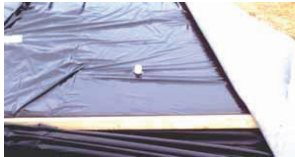
COMA-Meter installed in a newly cast airport runway slab for evaluation of the timing of cutting the joints.
