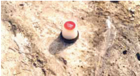
COMA-Meter installed in concrete for strength indication before stripping of forms in cold weather conditions.
