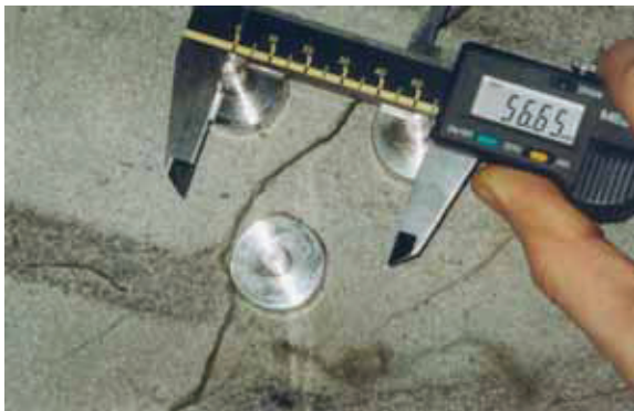
The CMD-200 being used for measurement of crack movement caused by ASR
