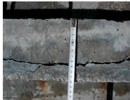
Figure 4. Cracks on the span beam
